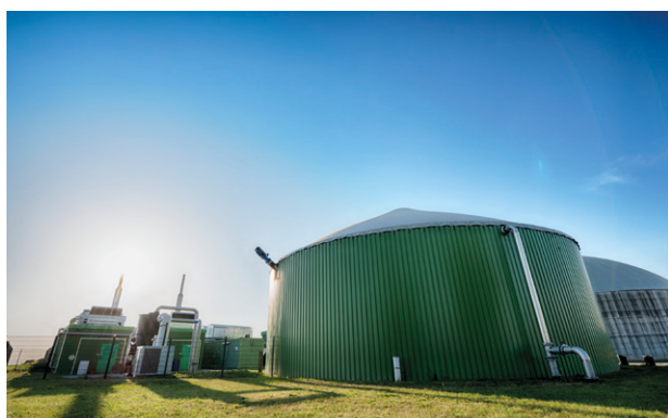
Biogas purification unit
